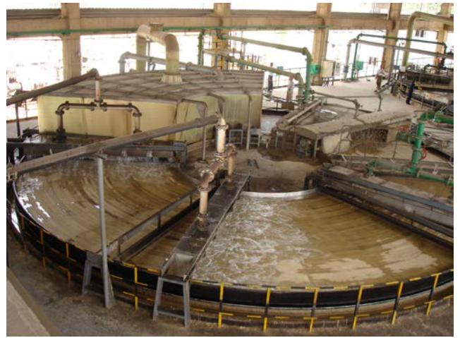
A HDZP filter operating in China in a P 2 O 5 Plant
