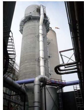
Ground level Candle Filter Vessel after Prilling Tower
